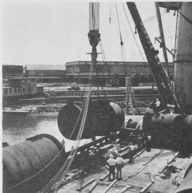
STACK SECTIONS were easily lifted off the freighter's deck and placed on a barge by the ship's crane. The Shunkoku Maru's deck crew wore safety hats.
